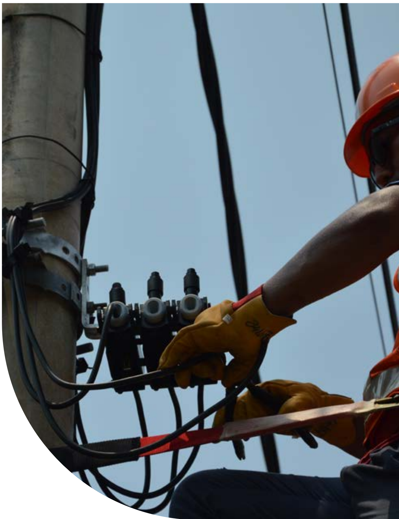
Fuse switch disconnecter MICHAUD installation - Tonga
